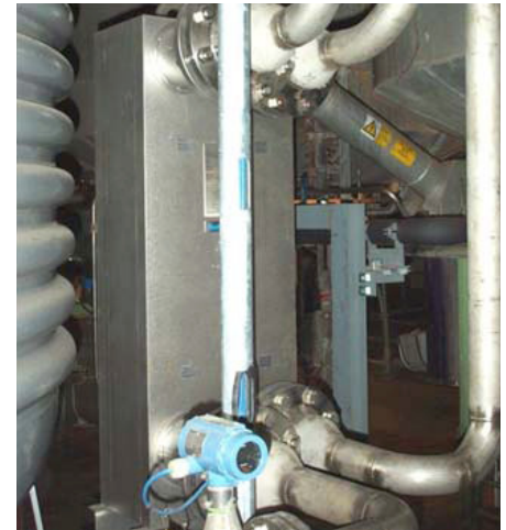
SIGMAWIG ST40 tempering of chemical reactor / Bayer Chemicals, Leverkusen
